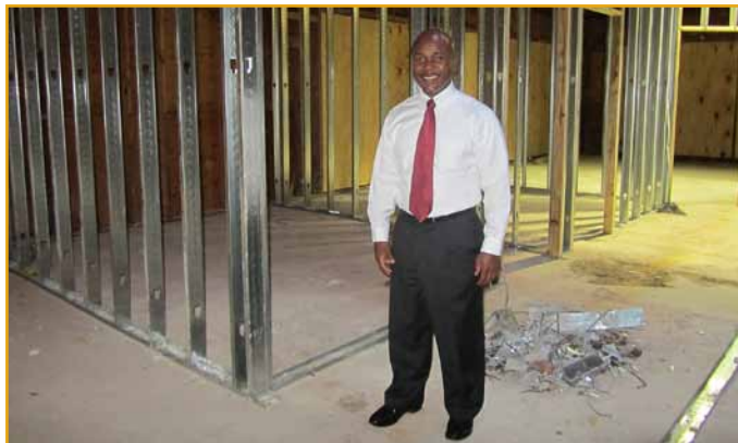
President Howe visits the construction site to monitor the renovations. Members can also view the progress of the renovation by visiting palmbeachbar.org/campaign.php
