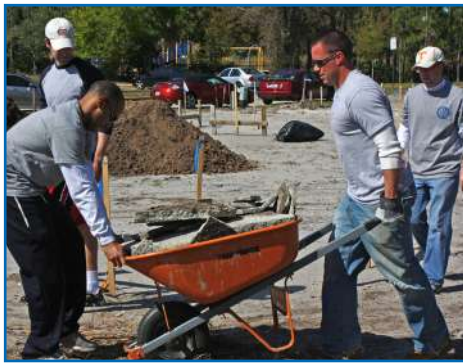
Nick Johnson, Tavis Souder, Collin White and Lee McElroy break concrete and haul it to a dumpster to prepare a new home site.
