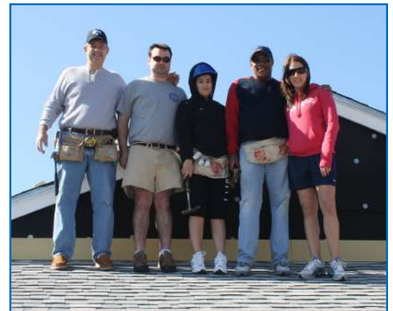
County Court Judge James Martz, Miles McGrane, the habitat homeowner, FL Bar Board of Governors Member David Prather and Julia Wyda work on applying wood to the side of the roof.
