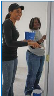
Tanya Reed and Rachel Johnson add the finishing touches to the paint inside one of the homes
