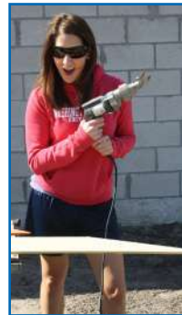
Julia Wyda uses power shears to trim down the siding that was applied to one of the homes.
